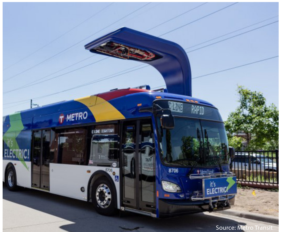
Figure 103: Transit electric charging station – C Line
