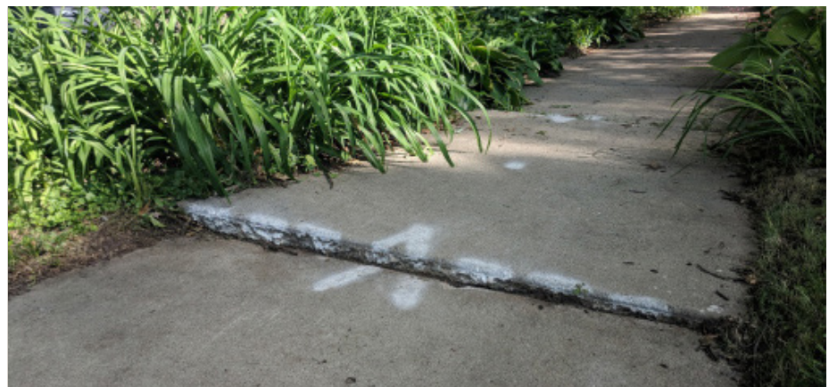
Figure 38: Sidewalk in need of replacement
