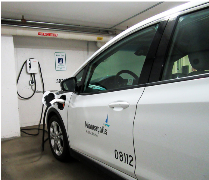
Figure 106: City of Minneapolis electric fleet
