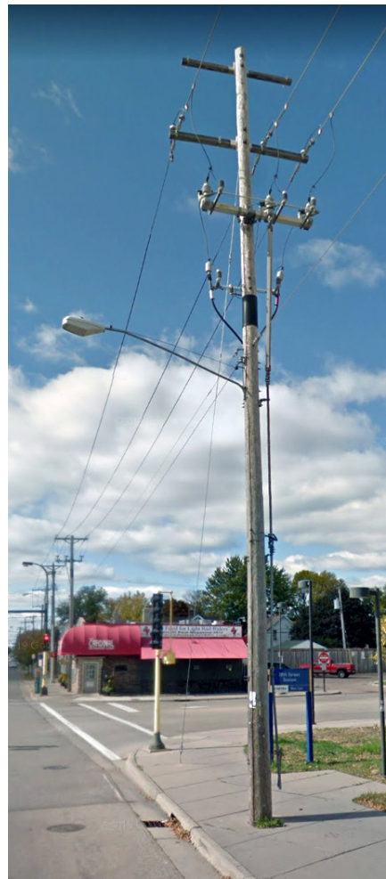
Figure 34: Wood pole streetlight
