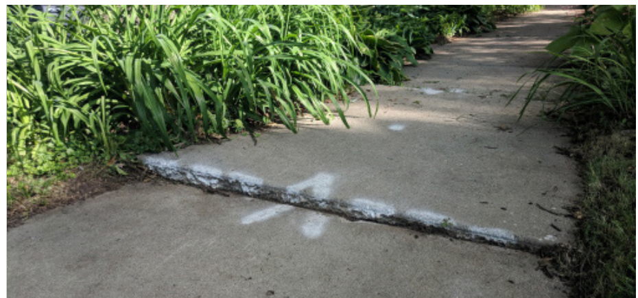
Figure 38: Sidewalk in need of replacement
