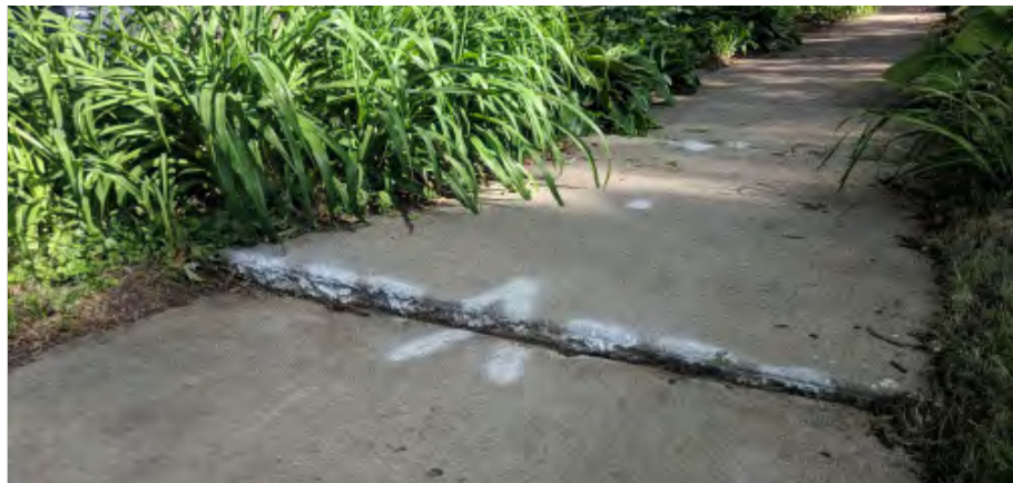
Figure 38: Sidewalk in need of replacement
