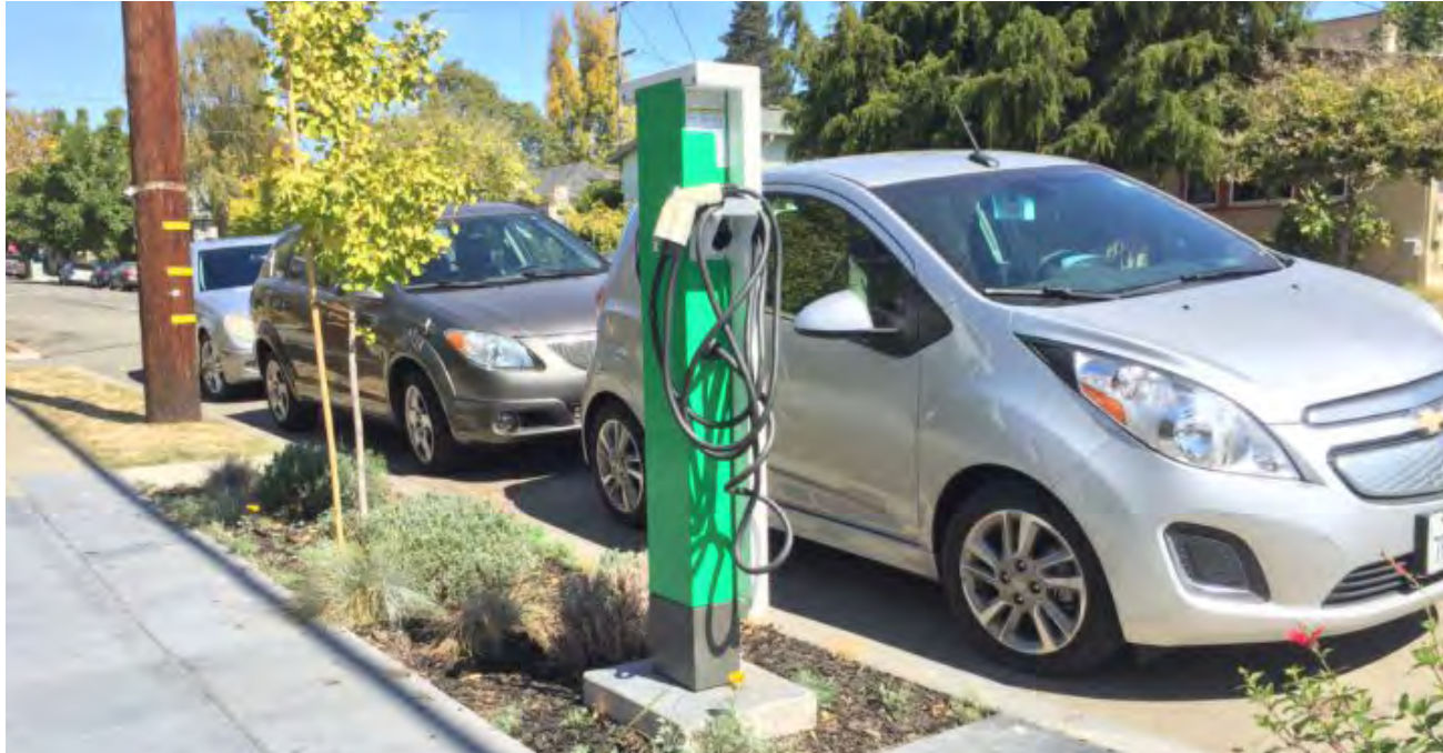
Figure 105: Electric vehicle charging stations in public right of way
