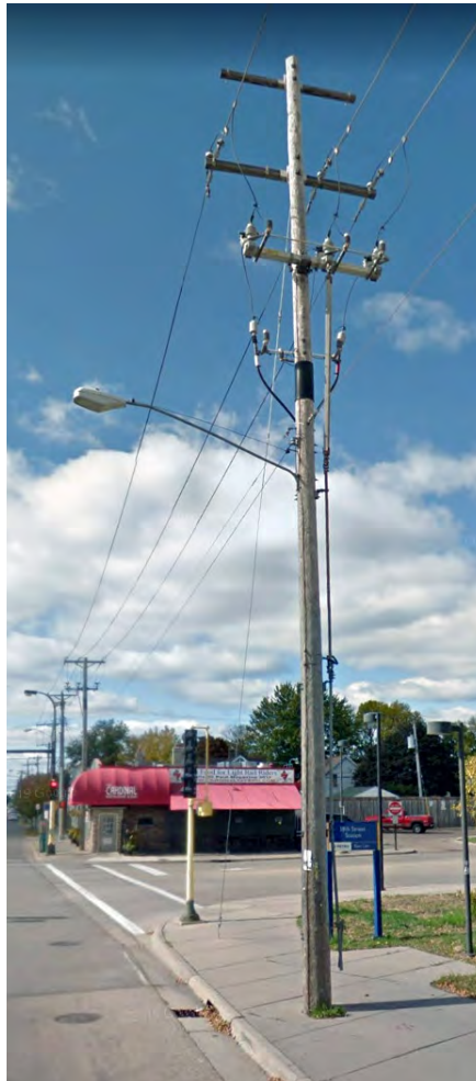
Figure 34: Wood pole streetlight
