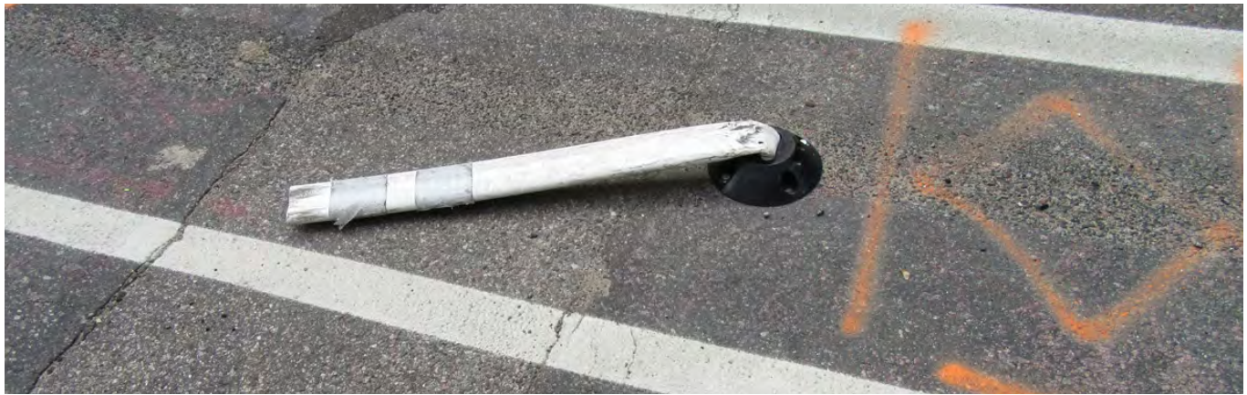
Figure 60: Bollard not maintained
